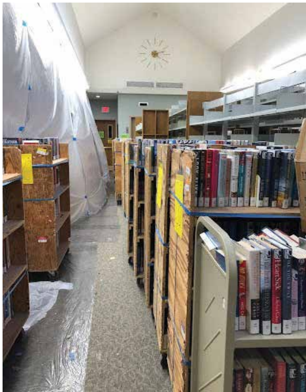
This photo shows the main floor of the Joshua Hyde Public Library under construction for an HVAC project, with carts full of books from the adult shelves. TURLEY PHOTOS BY ROWAN BERNSTEIN
