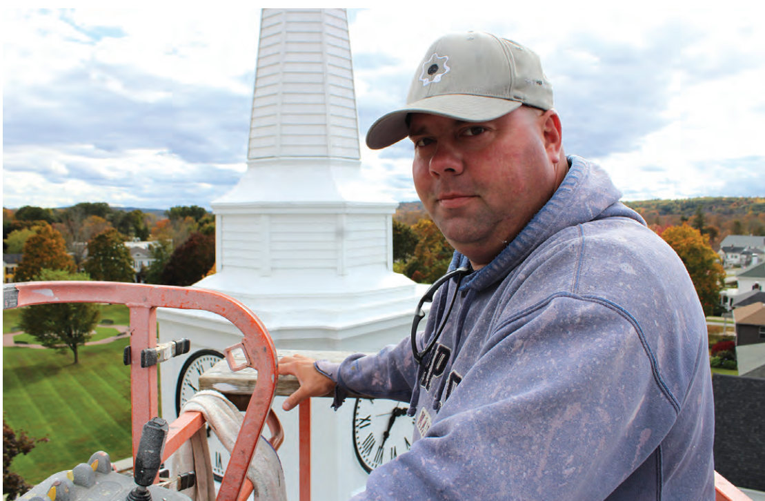
Chris O'Connor of Restco Corporation used his aerial lift to restore and paint the steeple and clock faces of the First Congregational Church of West Brookfield. TURLEY PHOTO BY PAULA OUIMETTE
