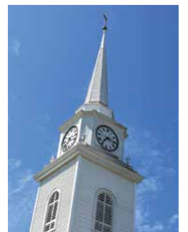
The steeple of the First Congregational Church of West Brookfield needs repairs. TURLEY PHOTO BY PAULA QUIMETTE
