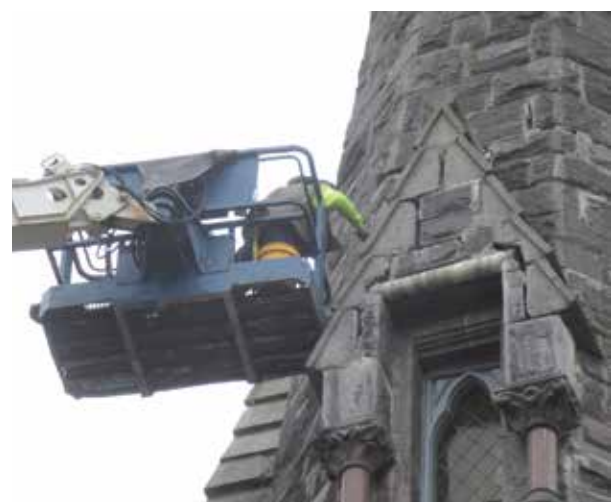
Workers are shown sealing lantern level exterior, which is necessary to keep new grout from seeping out of deteriorated masonry.
