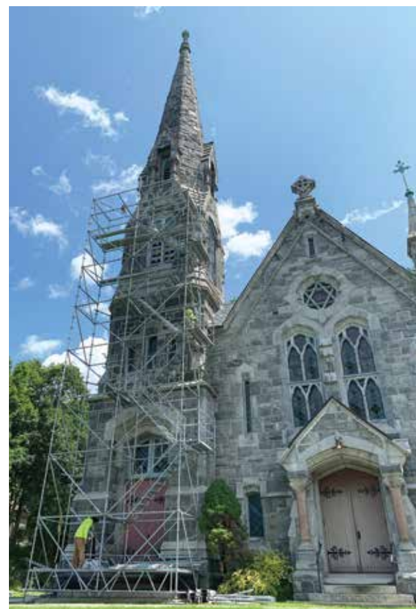
This photo shows the scaffolding at the Stone Church for Phase 4 Lantern Level interior stabilization. SUBMITTED PHOTOS
