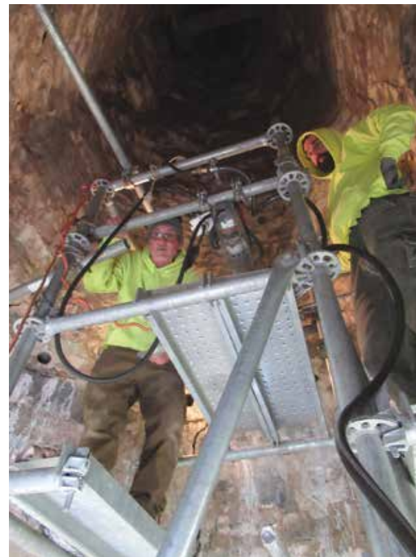
This shows the inside of the Stone Church job site at lantern level.
